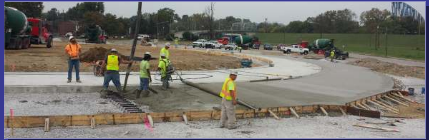
Above: Prus workers place another lane of the new concrete Roundabout near Newport.
