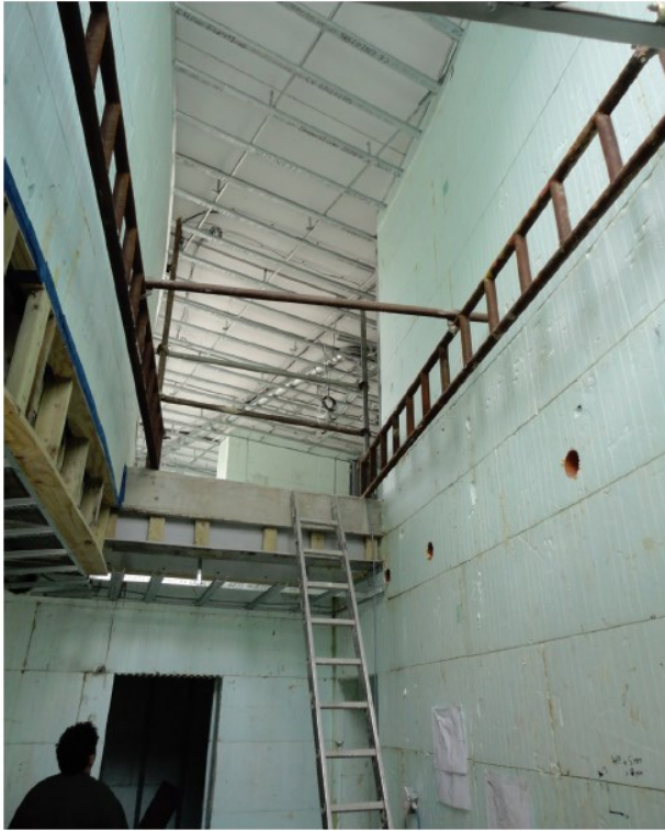
View of the unfinished interior of the Curly house after ICF walls have been completed.
