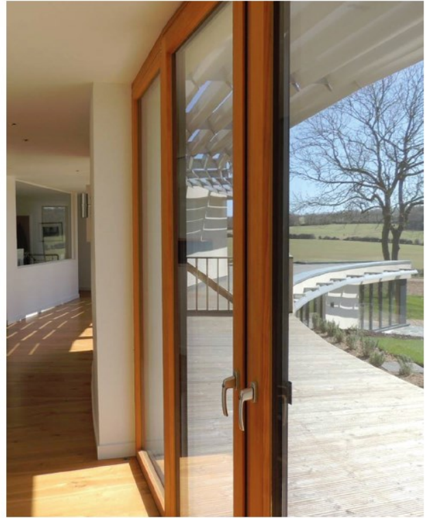
South facing high performance, triple-glazed windows manage heat gain.
