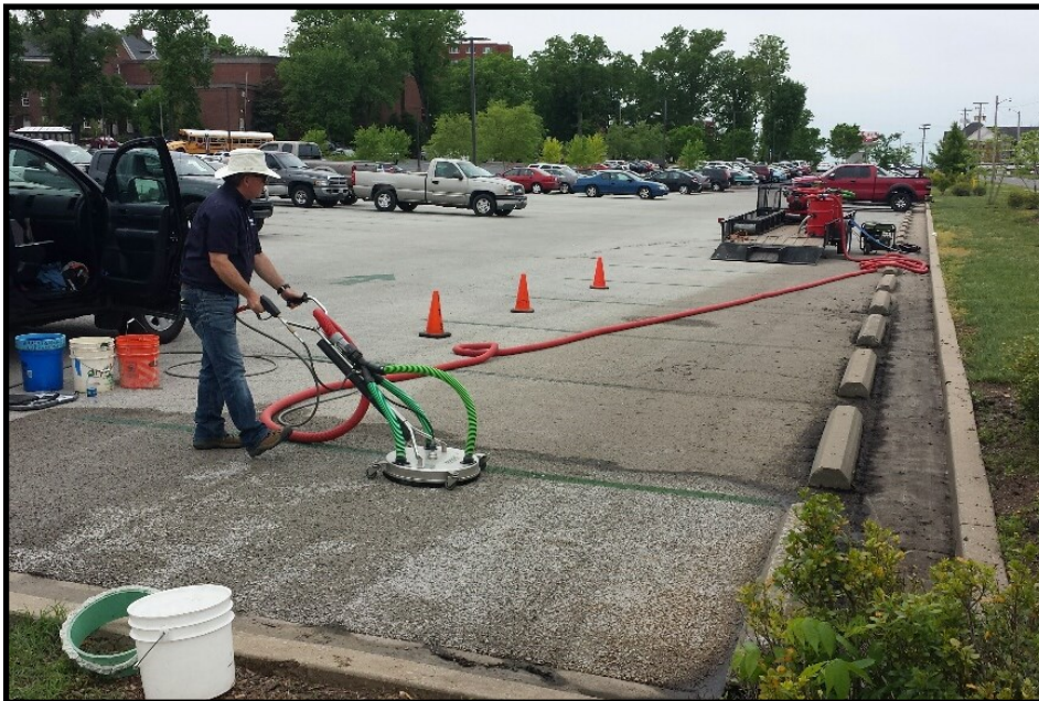
TCA Executive Director, Alan Sparkman, demonstrating the cleaning of pervious concrete at WKU.
